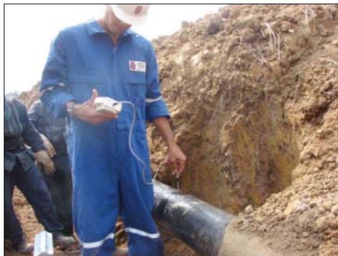
Technicians took manual measurements at four different points along the pipeline's circumference, starting at 12:00 and ending at 9:00 hr. The residual magnetic field measurement shown is taking place in the gap created by cutting the pipeline (Fig. 2).
